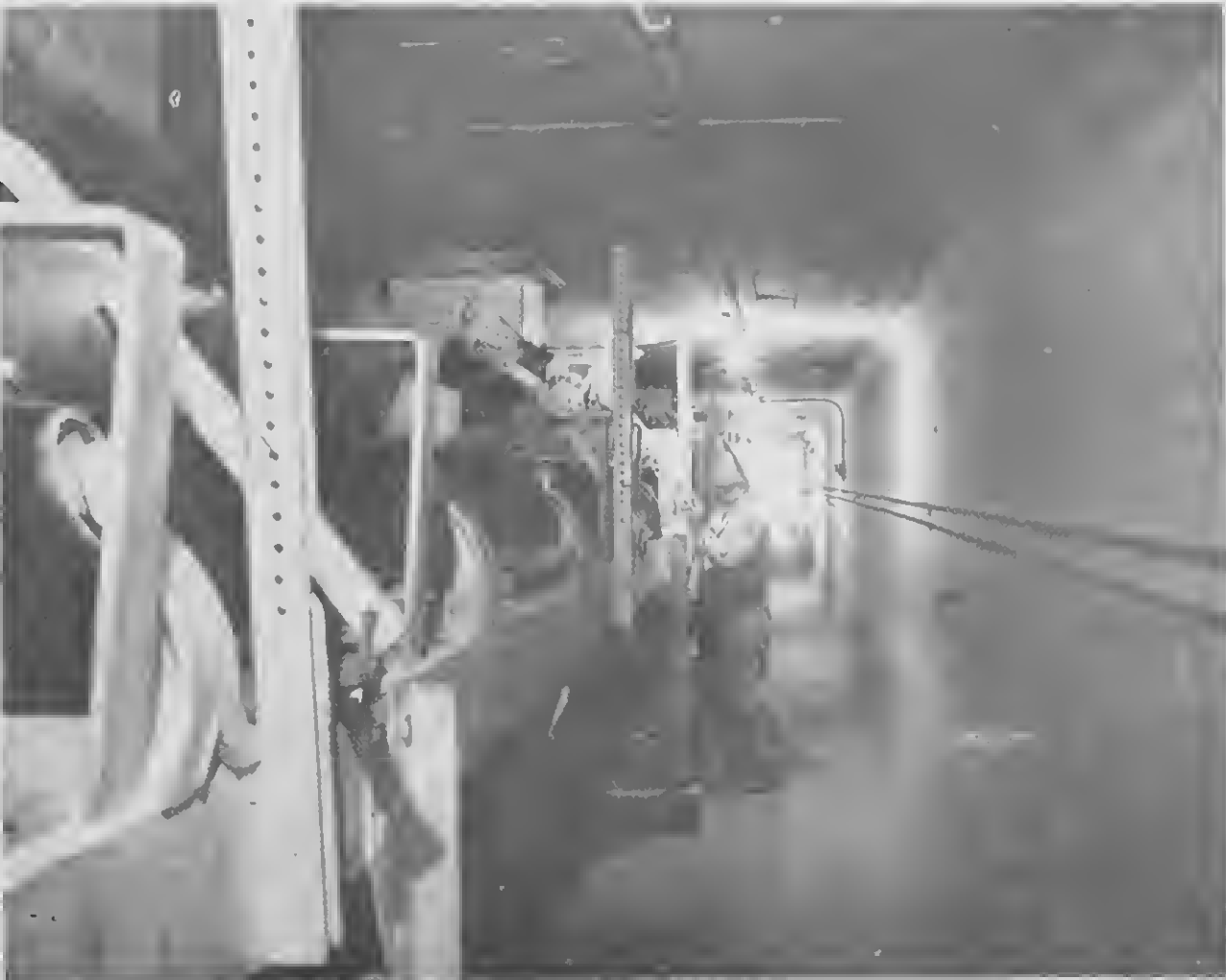
ARUBA'S ONLY tunnel stretches 50 feet underground below the storage piles in the picture above. The machinery at left controls the flow of materials from storage to use via conveyor.
